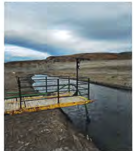
Emergency intake facility at the Oldman River Reservoir for nearby urban communities.
